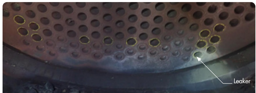
(b) Tube-to-tube sheet joint leak at location of high stresses predicted by FEA
