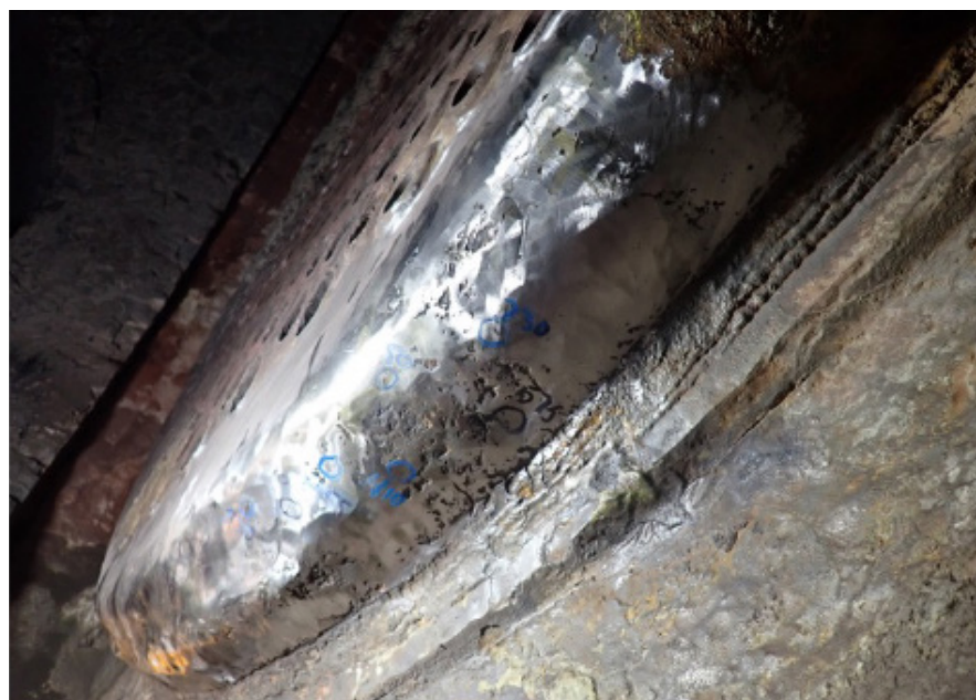
(b) Tube sheet repair at the bottom leak location
