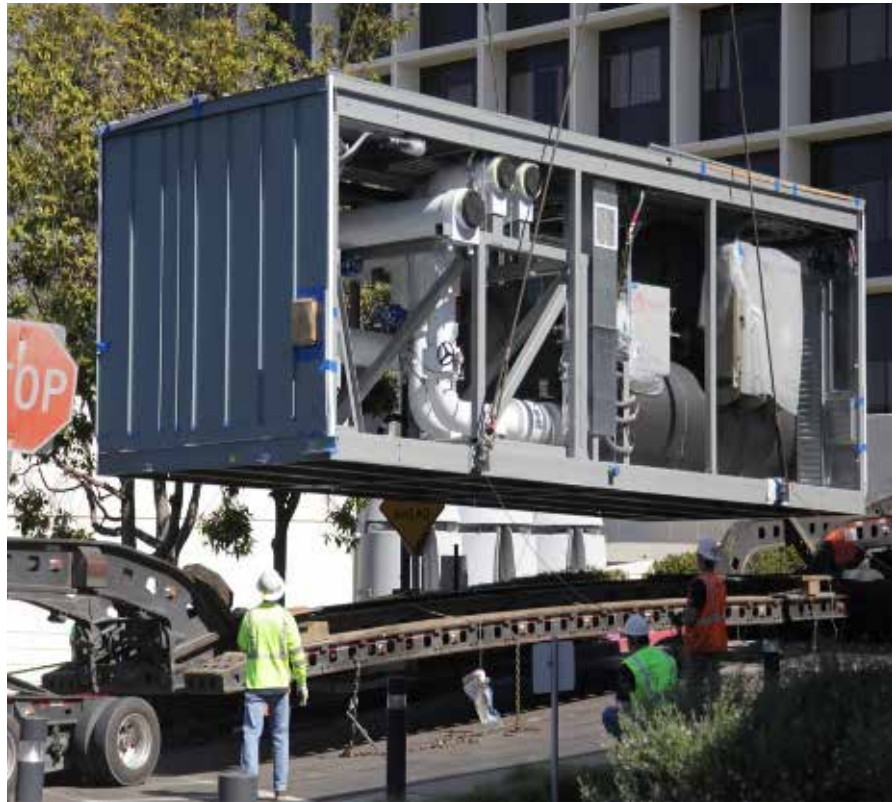
FIGURE 1. Lifting of Modular Central utility plant at Scripps Green Hospital, San Diego, California
