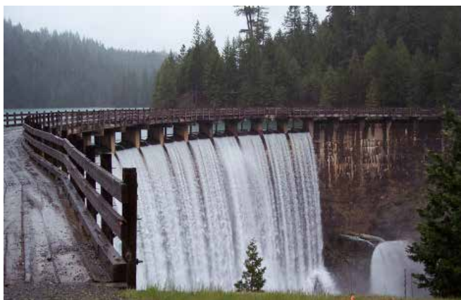
FIGURE 2. Concrete arch dam circa 1909, aging degradation Issues subject to increased flood and seismic demands
